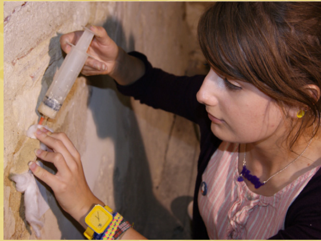
Above: Grouting behind existing layers of lime wash in the West wall to restore stability to the heavily restored area
