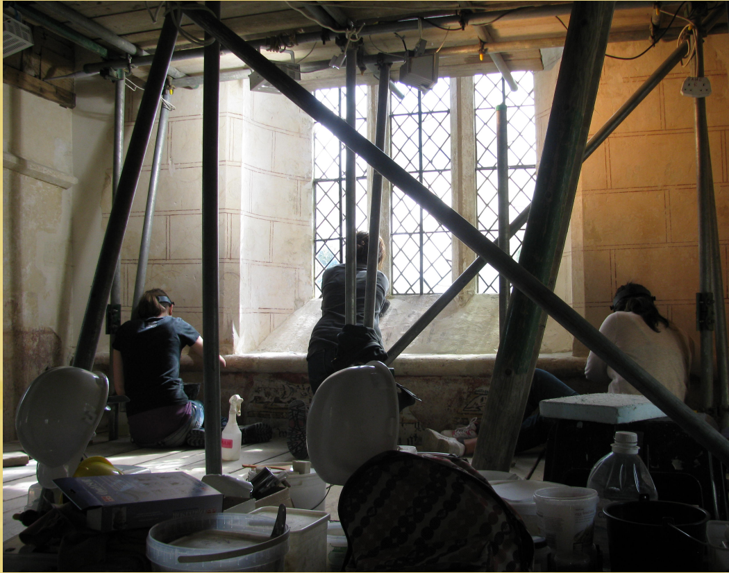
Above: Three volunteers (HC on far left) conducting wax reduction and gap filling treatments in the Chancel
